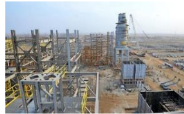
Jazan Gasification Plant
